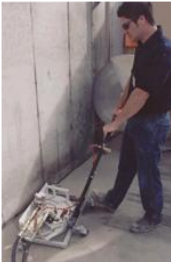
For making the flush cut along the floor, a flush cut hand saw on a cart could be used instead of a flush cut wall saw.
